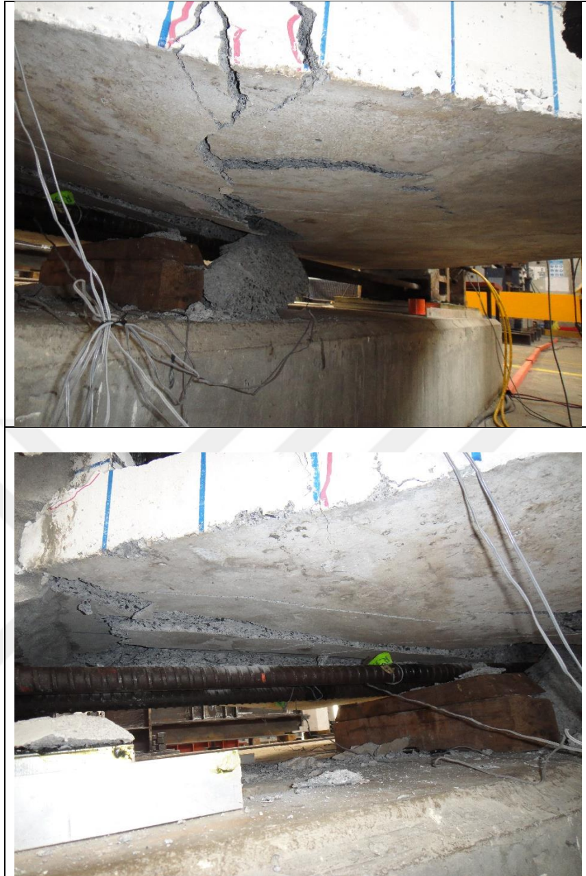
Figure 3.20 : The bottom cracks of the voided slab.
